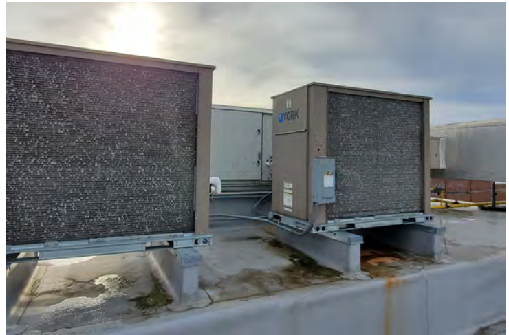
Pool dehumidification system
